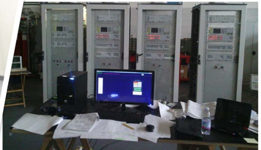
F&G Panels for Stogit Compressor Station
