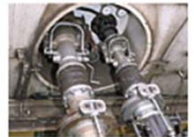
Fuel Loading Racks
